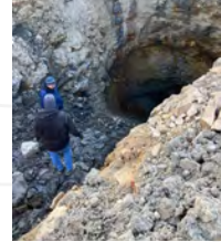
Recovery Division Biologist Greg Turner and machine operator inspect a vent bore hole after creation.
